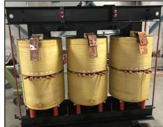
Top clamps and new insulators installed and then sprayed with dielectric varnish
