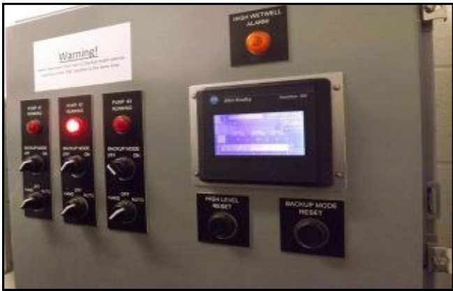
Turn key solutions with custom fabrication
